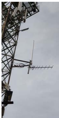
Figure 1 – VHF antennas of the BSDC transmitting complex on the Control's room antenna mast
