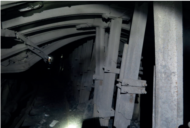
Figure 1 – Deformation of the metal arch support with changing the rock pressure
